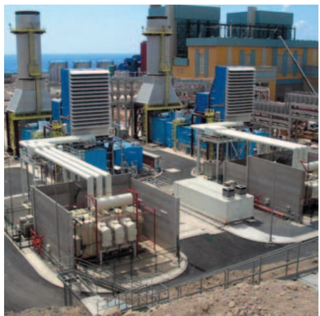
Combined-cycle power station in Granadilla (Tenerife)
