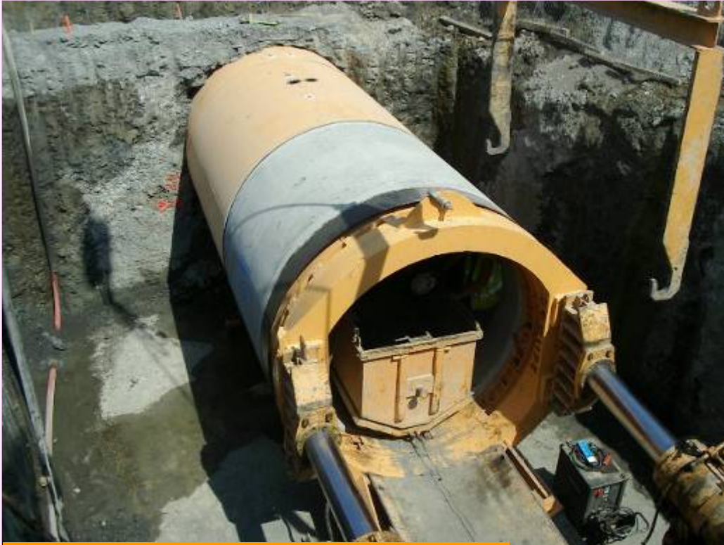
220kV underground system
