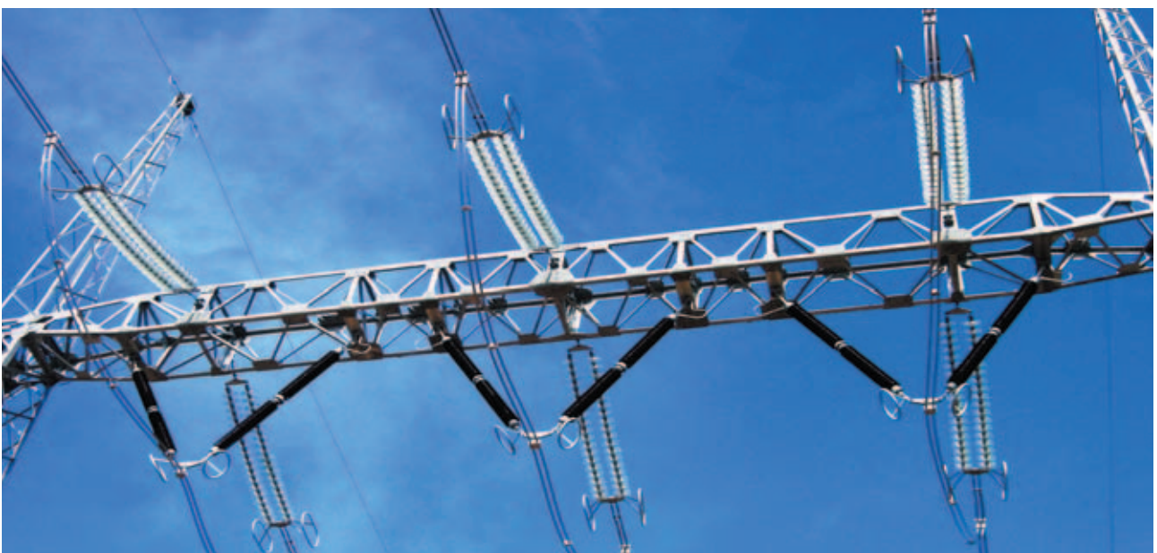
High-voltage electrical grid
