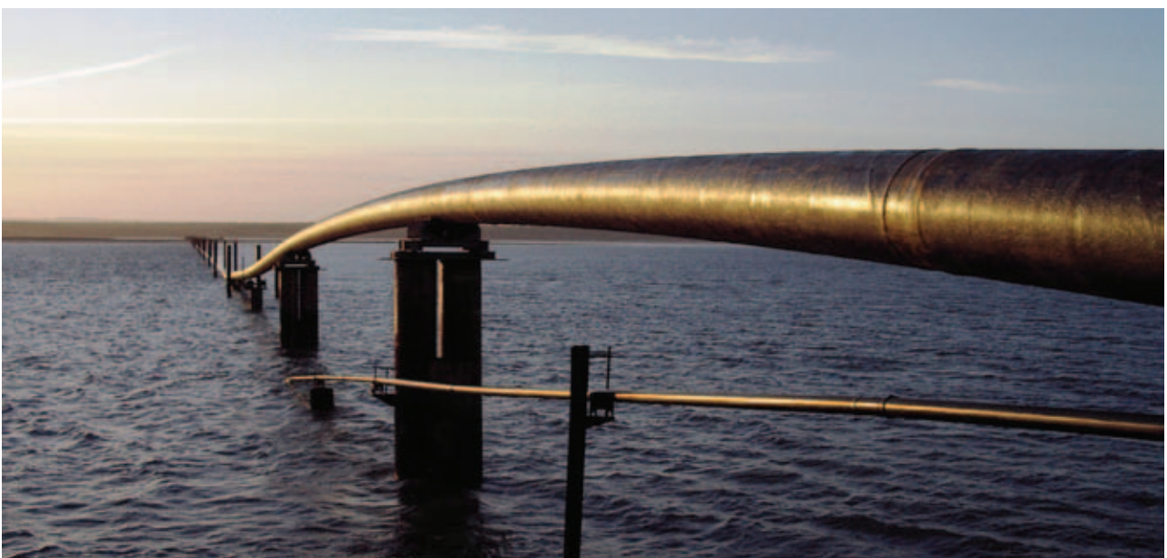
Sines-Setúbal gas pipeline (Portugal)
