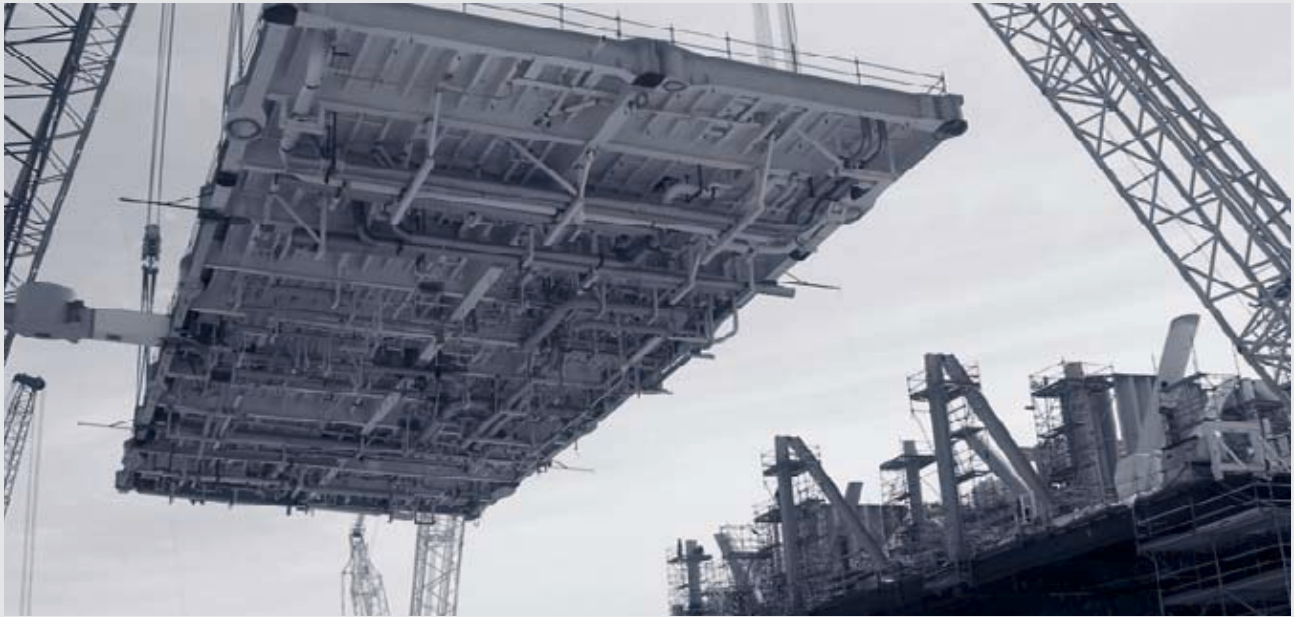
Buzzard Project in the North Sea
